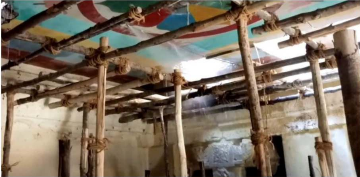
Before Thiruppani; Concrete ceiling in RajaGopuram
